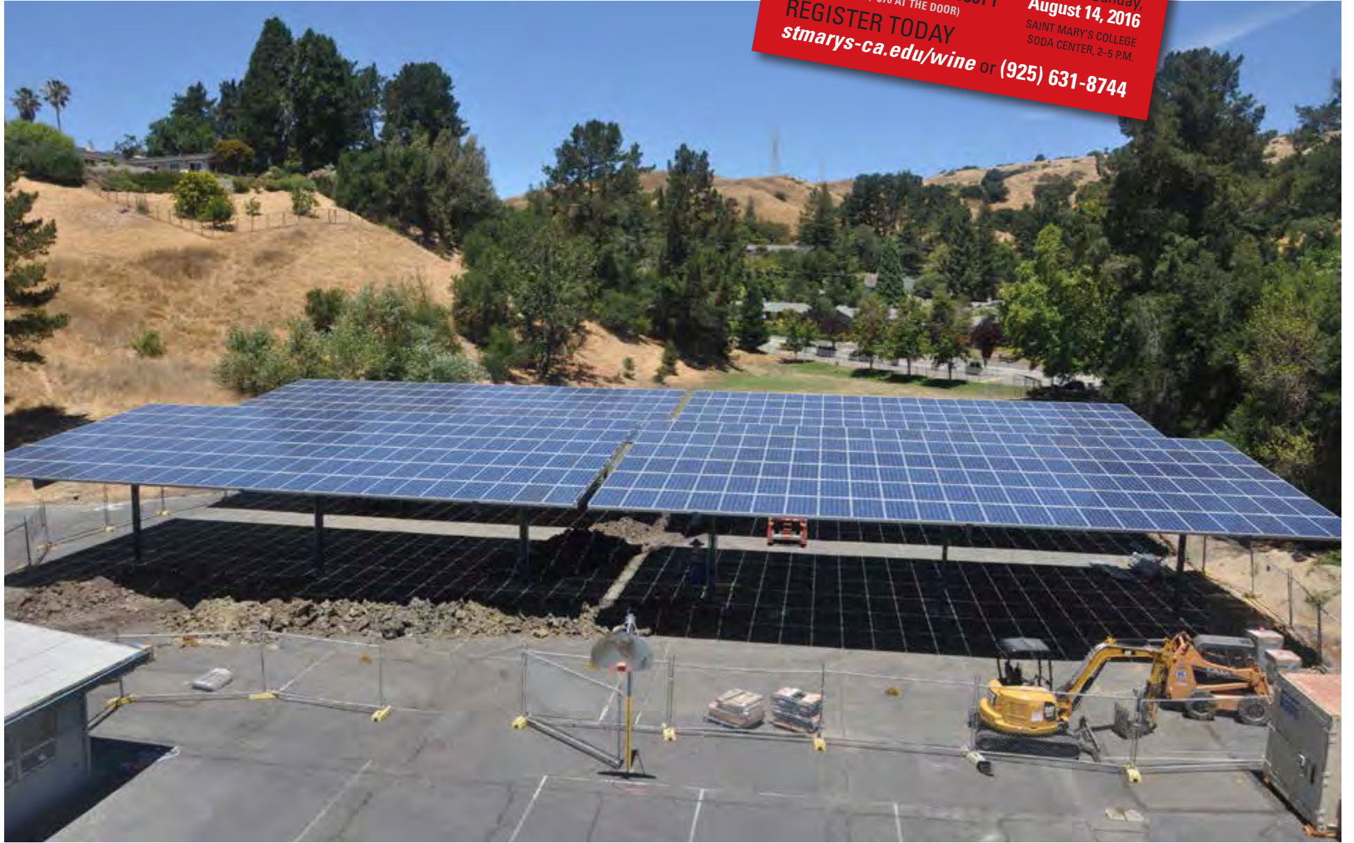
Solar panels are being installed at Orinda Intermediate School, above, as well as at all OUSD elementary schools and at Lamorinda high schools.
